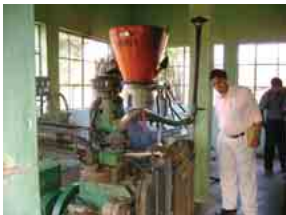
Biomass based power gasifier operating in Mahishakada village, Orissa
