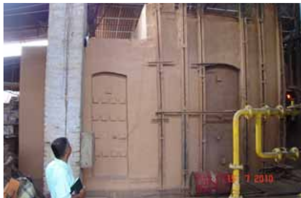
Regenerator in a tank furnace unit
